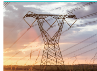
Power Grid System
